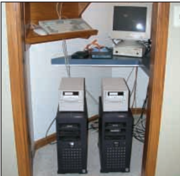
Fig. 5 Dedicated server closet in Dr. Way's office.
